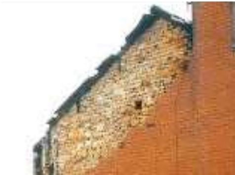
An extreme case of wall tie failure!
