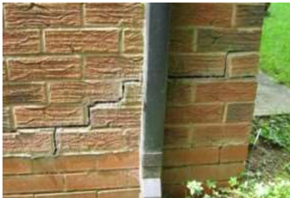
Some examples of cracking caused by subsidence
